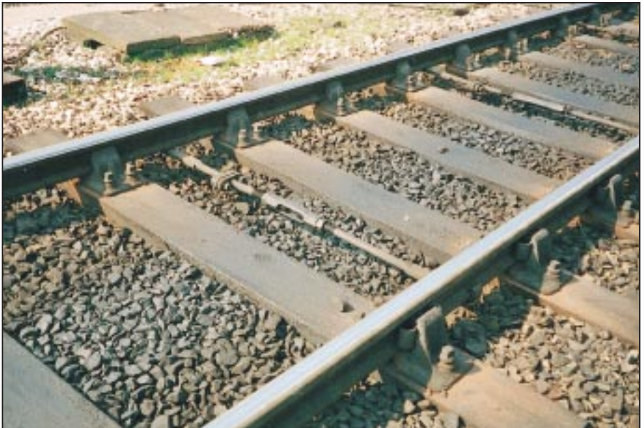
Figure 13 Tie bars must be checked on each track inspection
