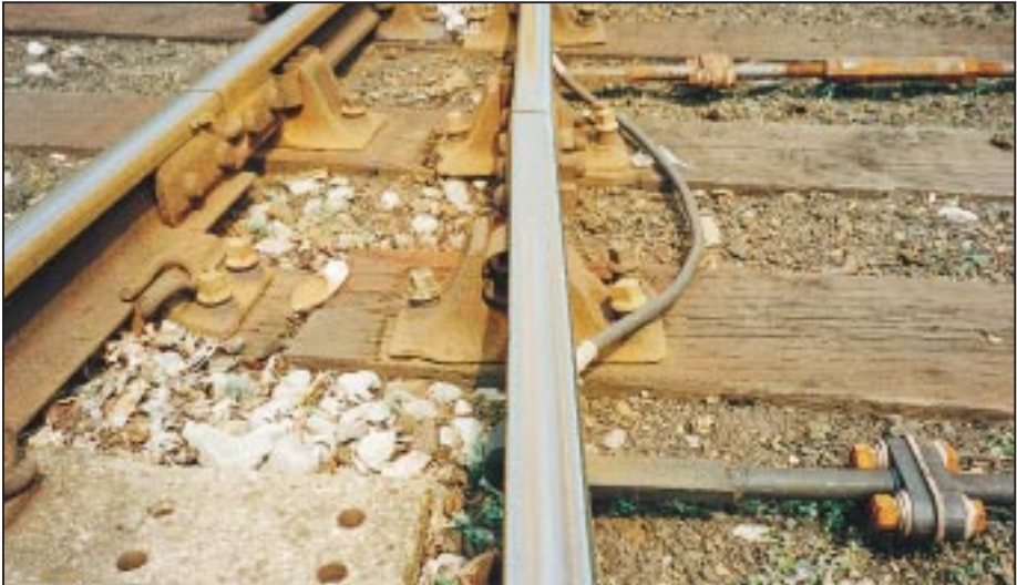
Figure 12 Leaning chairscrews in this S&C indicate gauge spread
