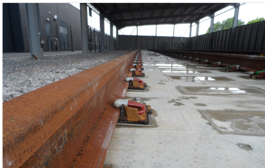
Image 4: Baseplates installed at Doncaster High Speed College waiting for decay rate measurements carried out by ISVR
